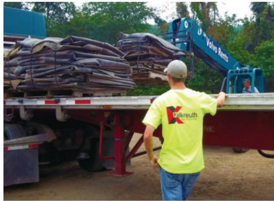
A Kalkreuth Roofing & Sheet Metal employee loads stacks of EPDM from Brooke High School onto a truck for transport to the recycler.
