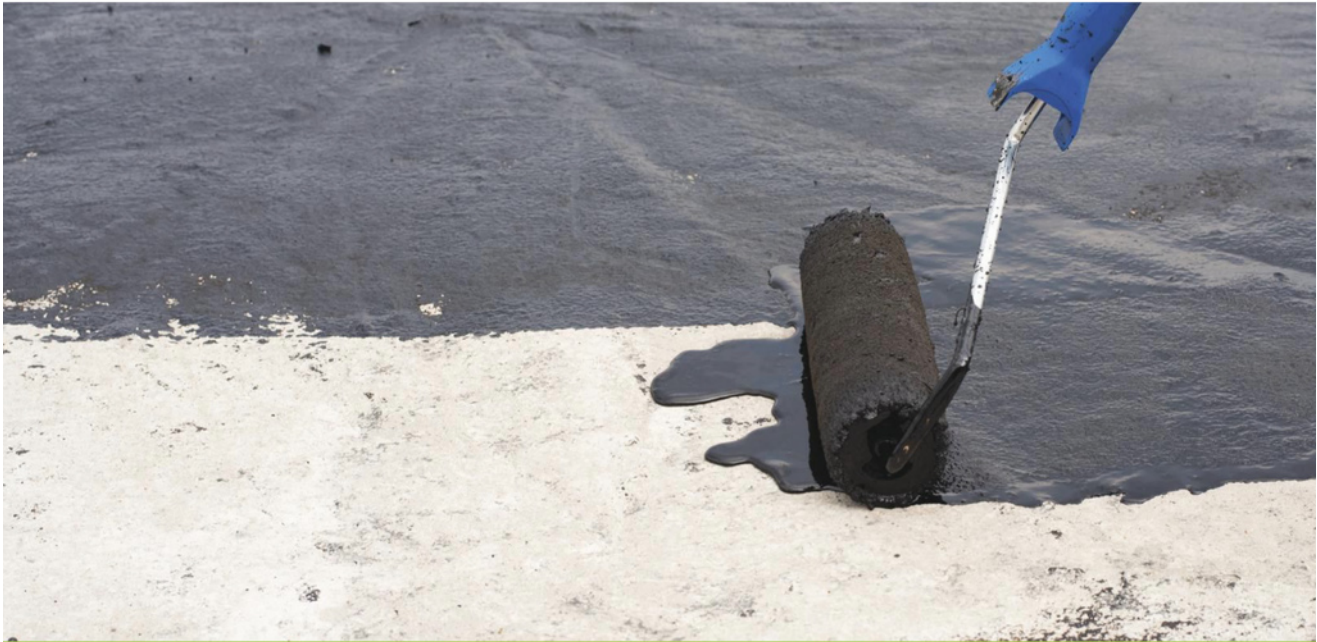
:: Roof coatings have evolved into a credible alternative that can go toe-to-toe with any low-slope system.
